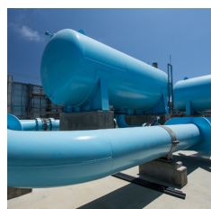
Claude "Bud" Lewis Desalination Plant in Carlsbad
