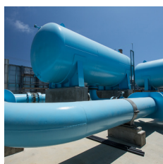
Claude "Bud" Lewis Desalination Plant in Carlsbad
