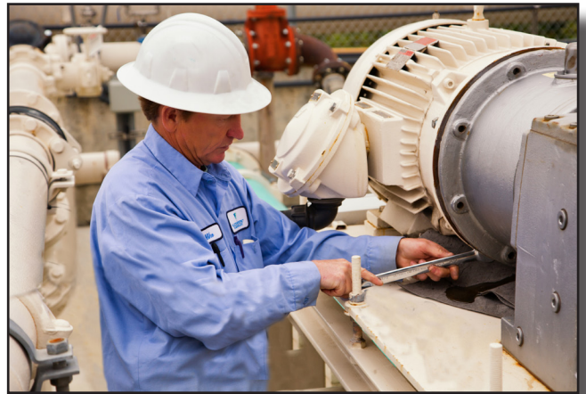
Staff work diligently to maintain the District's extensive assets, including this pump at the Meadowlark Water Reclamation Facility.
