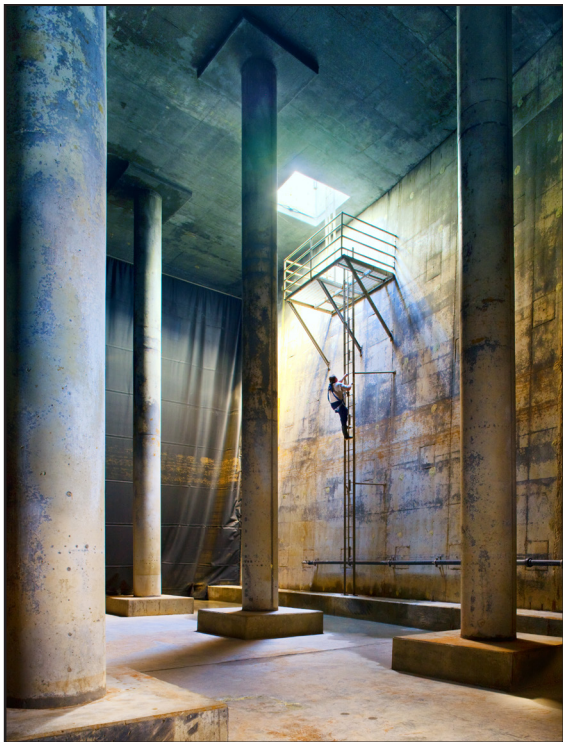
Inside the District's 33-million gallon Twin Oaks Reservoir, one of the largest pre-stressed concrete tanks in the world.
