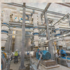
Claude "Bud" Lewis Desalination Plant in Carlsbad
