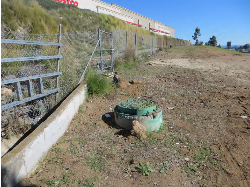
Photograph 2: Standing at the western end of the project facing east at one of the two manholes marking the access points along the western terminus.
