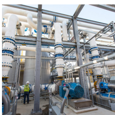
Claude "Bud" Lewis Desalination Plant in Carlsbad
