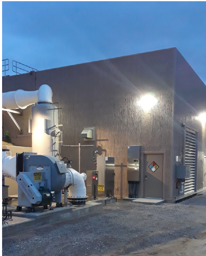
Agua Hedionda Pump Station
