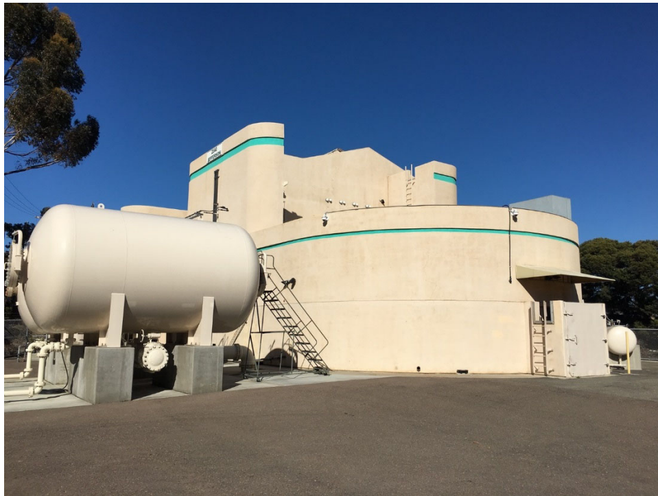
Buena Vista Pump Station
