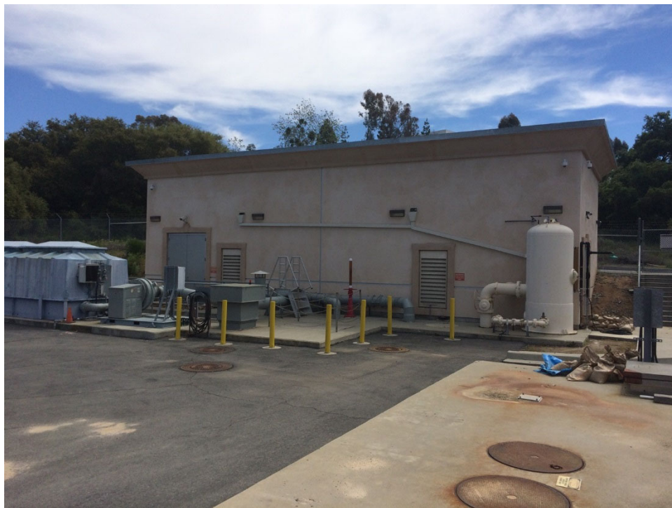
Buena Creek Pump Station
