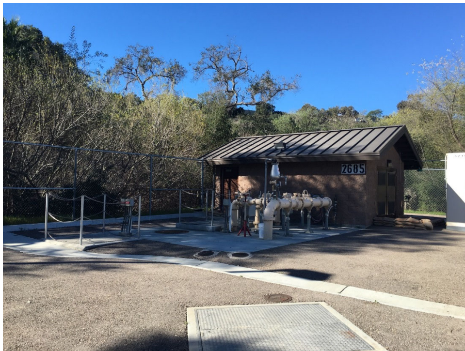
Raceway Basin Pump Station
