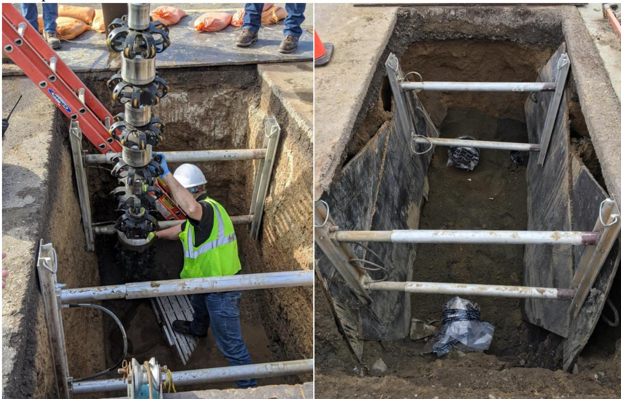
Figure 5: 12” WHG access pits – Left: launch pit near the Hampton Glen intersection with the 12” SeeSnake tool being lowered for insertion into the line; right: retrieve pit near the Palos Vista Reservoir tank prior to setting up the winch line.
