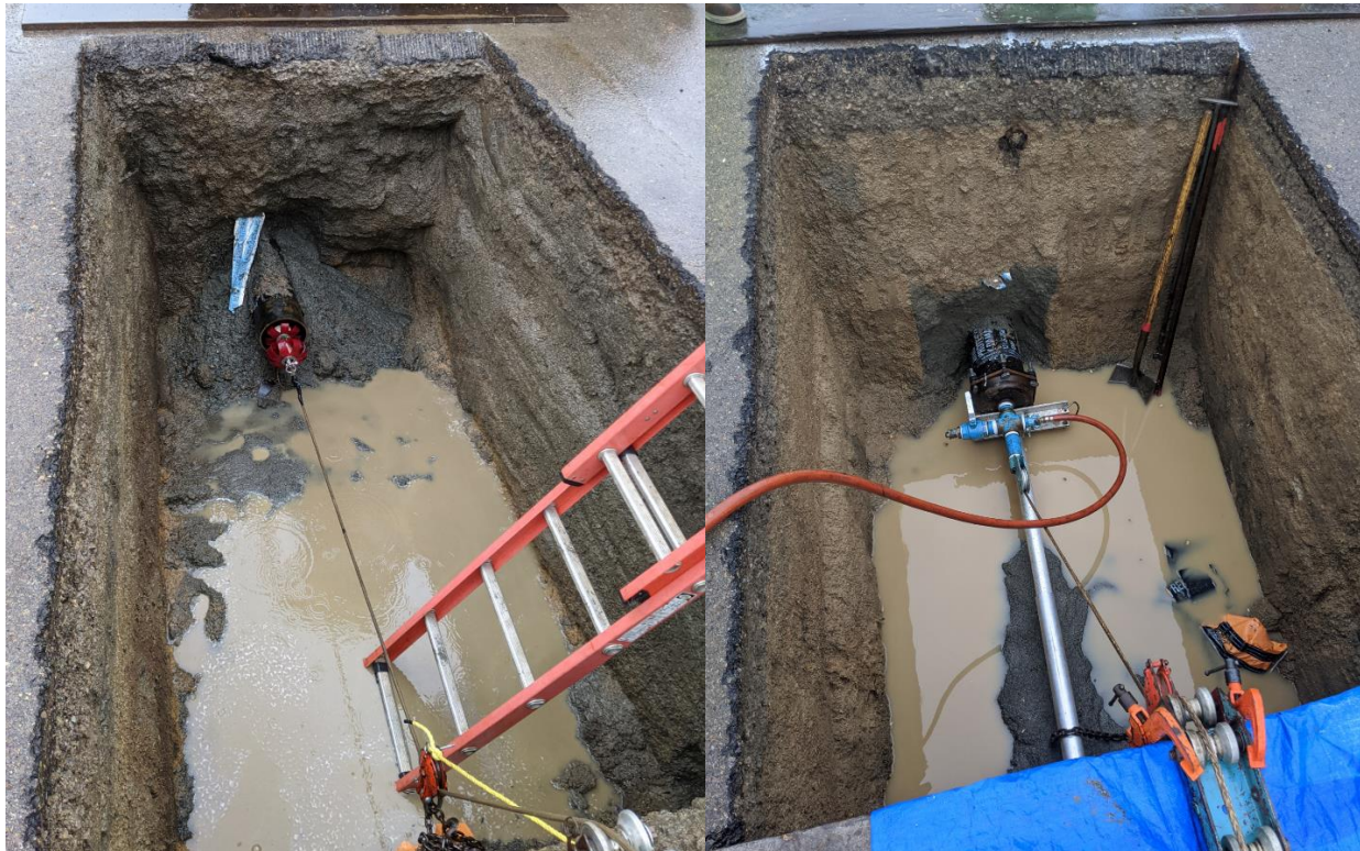
Figure 4: 8” KG access pits – Left: launch pit near the Hampton Glen intersection with the 8” SeeSnake visible just before commencing the 706ft run between both access pits; right: retrieve pit at the southeast end of Kensington Glen. as the 8” SeeSnake is being pulled through the line for the RFT inspection.
