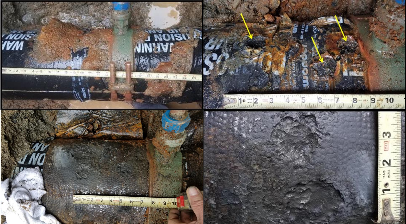
Figure B1: Verification photos of AOI #2 - Pipe 0690, 26% remaining wall (10:30) at 1149.63ft. To the right of the corrosion patch is a collar for a service connection. All photos are courtesy of RFYeager Engineering.
