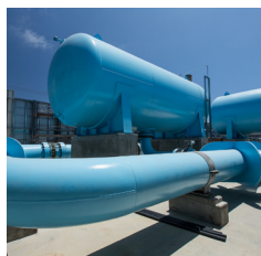
Claude "Bud" Lewis Desalination Plant in Carlsbad
