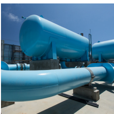
Claude "Bud" Lewis Desalination Plant in Carlsbad
