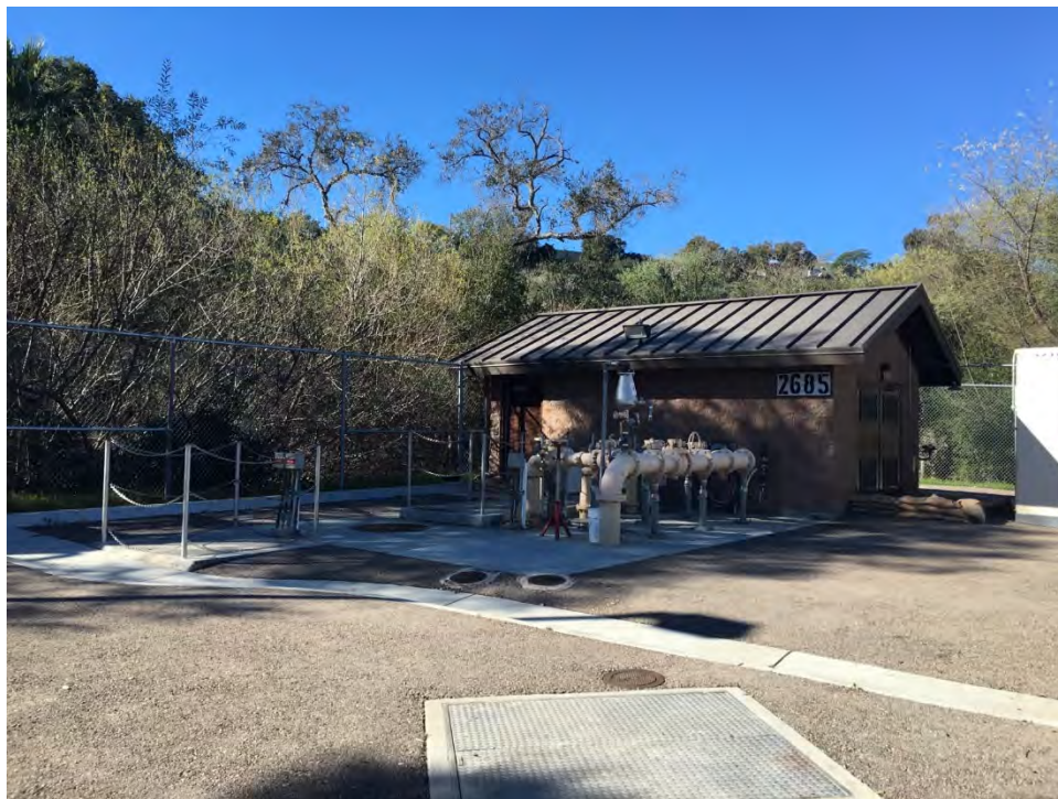
Raceway Basin Pump Station
