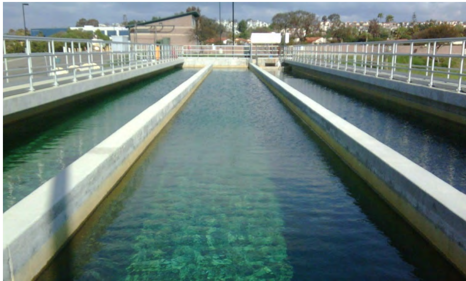
Carlsbad Water Recycling Facility
