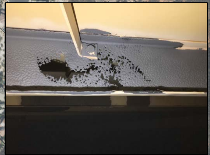
BLAST INSPECTION - CORRODED RAFTER
