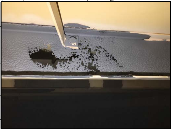
BLAST INSPECTION - CORRODED RAFTER
