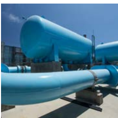
Claude "Bud" Lewis Desalination Plant in Carlsbad
