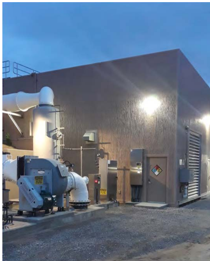
Newly Constructed Agua Hedionda Pump Station
