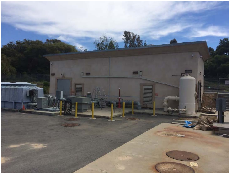
Buena Creek Pump Station
