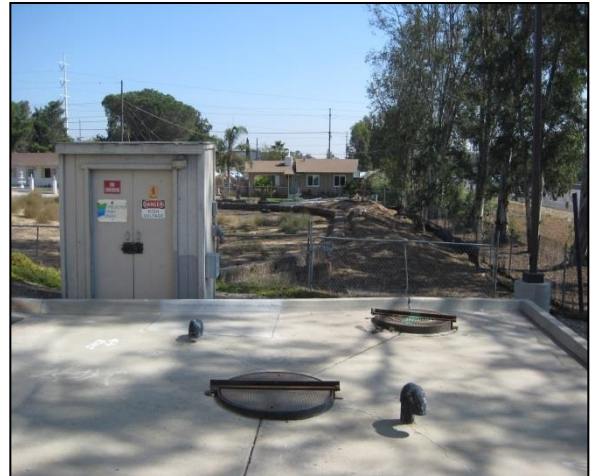
The Montiel Lift Station is the District's smallest lift station.
