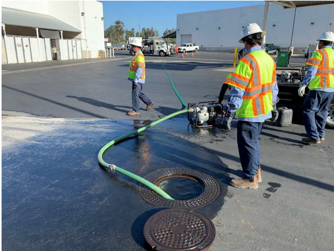
Figure 6: Simulated Pump Around & Draining of the Training Center Manhole
